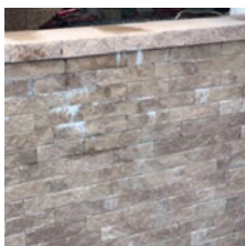
Mineral deposits on a wall installation
